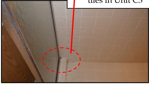
Cracked/separated tiles in Unit C3
