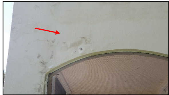
Bubbles behind paint are indications of water intruding the wall above.
