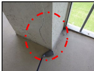
Cracked column on balcony.
